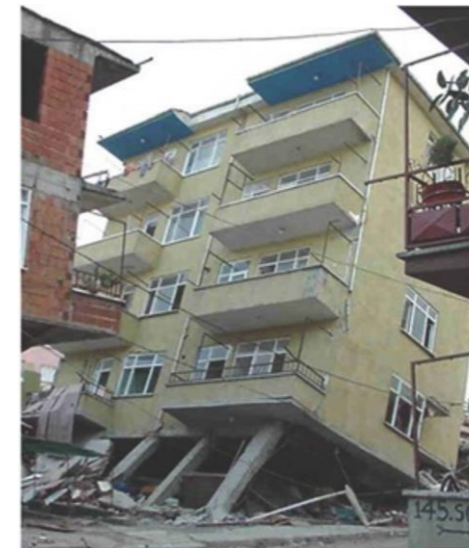
Soft story failure
