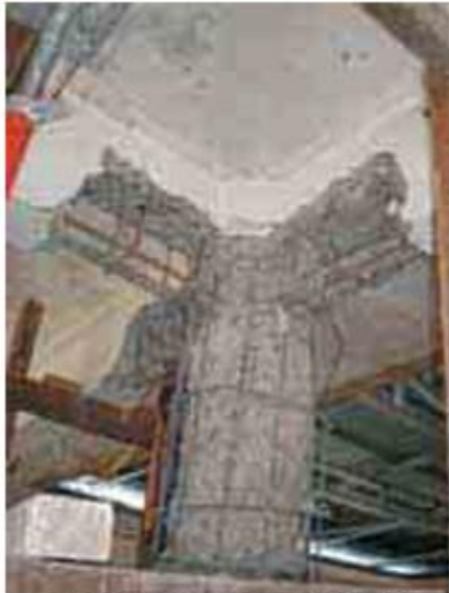
DAMAGED COLUMN, STIRRUPS & ANCHORING ARE NOT ADEQUATE
